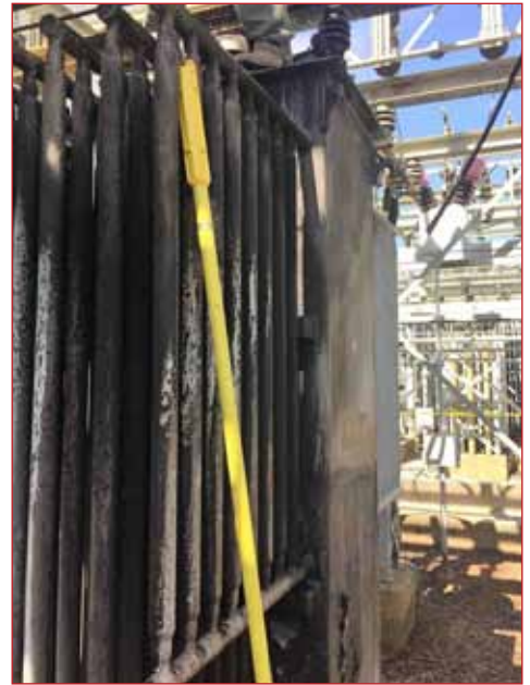
Damaged Station Service Transformer
