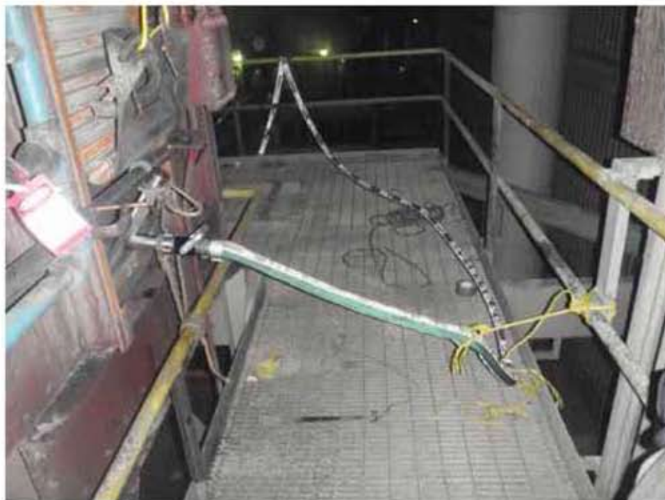
Hazard mitigation equipment tied up and secured for remote activation.
